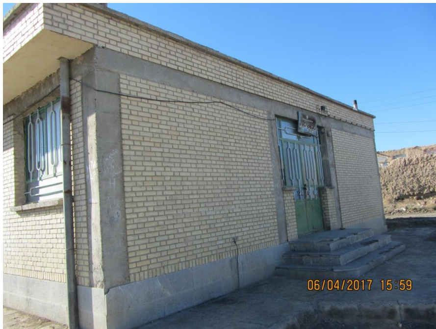
Figure 8. No damage to the Alghur village school building, which has been built in compliance with the principles of earthquake resistance design.
