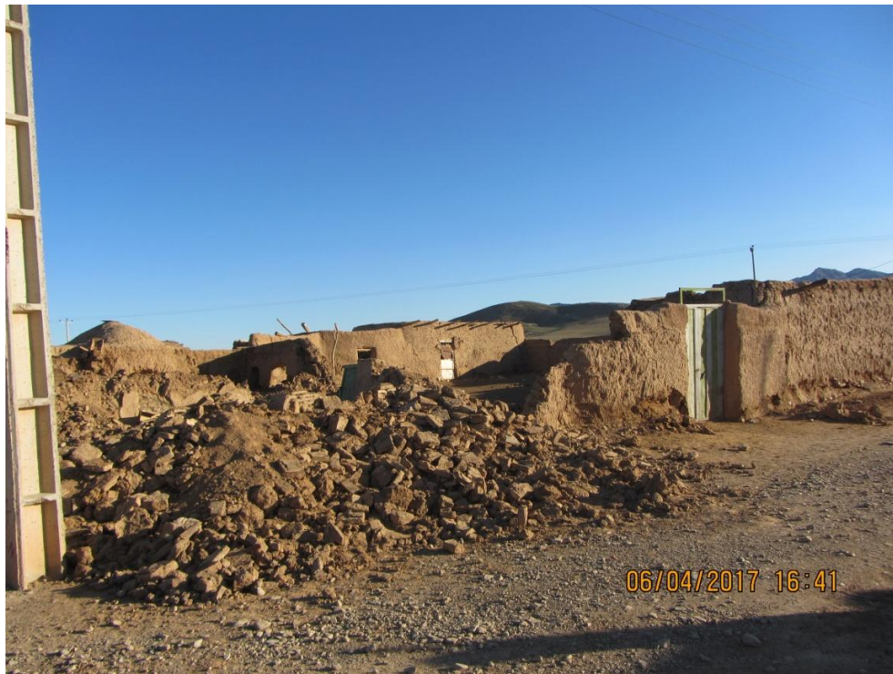
Figure 11. Collapse of the walls and demolition of the farmhouse in Ghale'e-Sorkh village.
