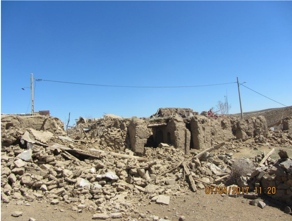
Figure 12. Destroyed farmhouse in the Kalateh-Ghadam village.
